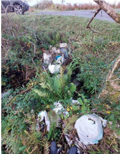
Rubbish dump at southern culvert of identified WCC4 27/10/2022.
